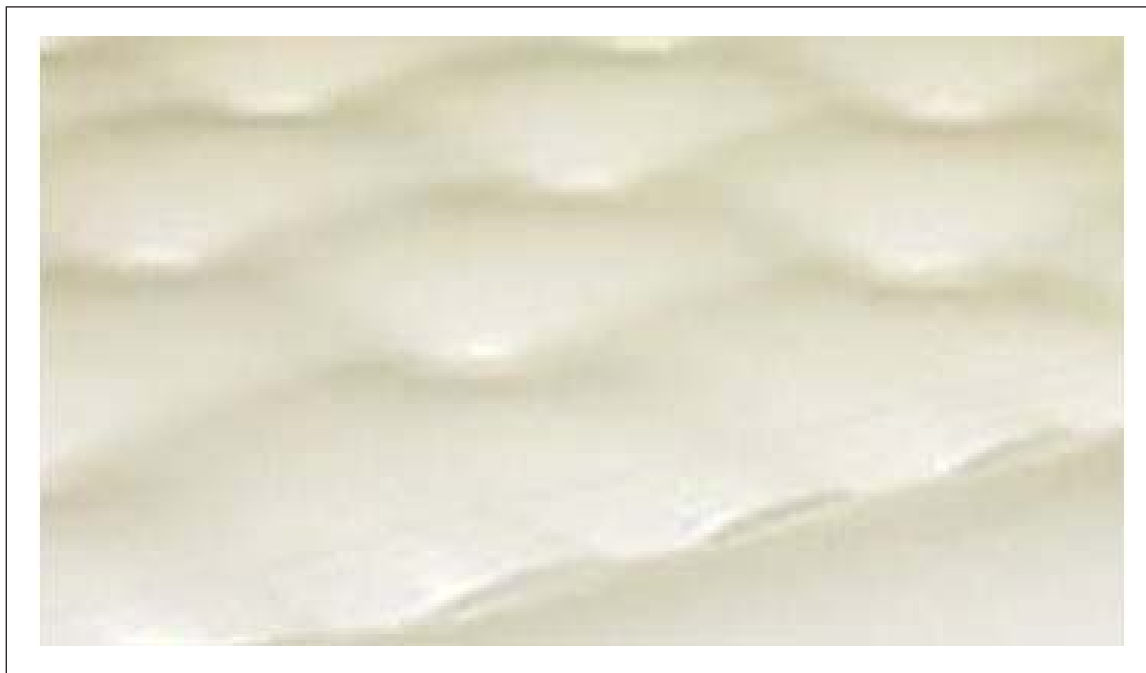
Fig. 7. Mechanically fastened roof cover billowing when subjected to wind pressure
