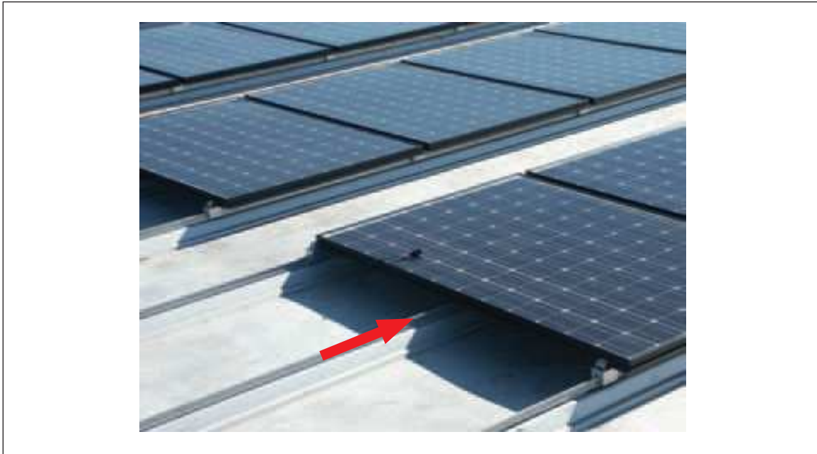
Fig. 11. Unacceptable arrangement: clamp missing from SSR rib below middle of outer panel edge
