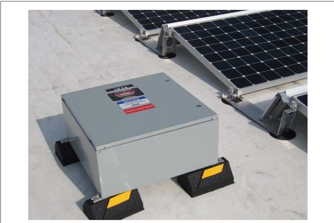
Fig. 9. Equipment lacking anchorage to roof framing
