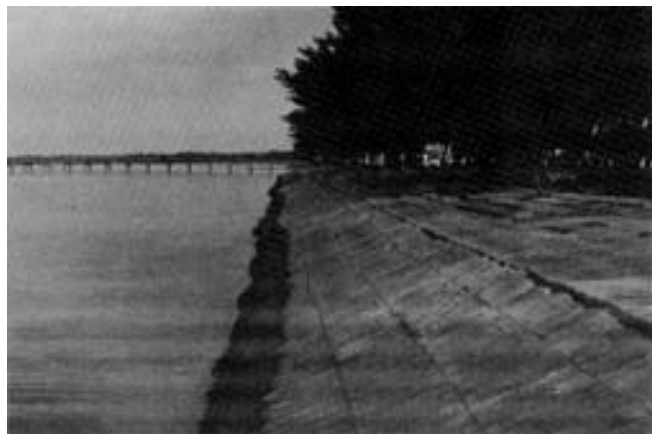
Figure B-28. Lok-Gard block revetment, Jensen Beach Causeway, FL
