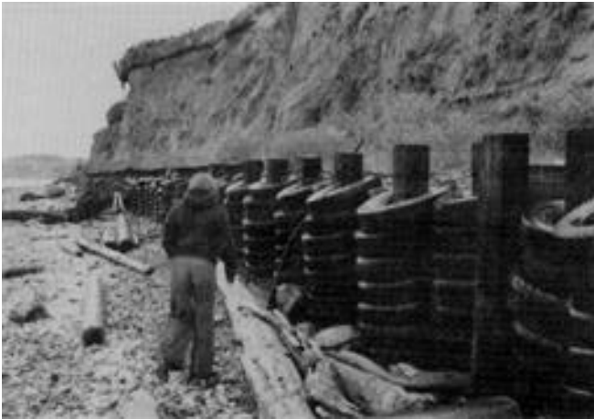
Figure D-18. Used rubber tire and timber post bulkhead, Oak Harbor, WA
