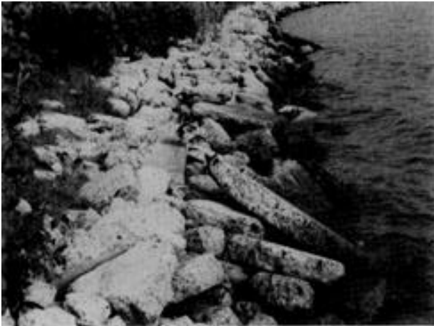
Figure B-7. Broken concrete revetment at Shore Acres, TX
