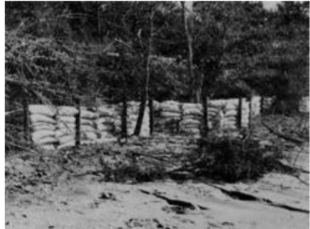
Figure D-16. Hogwire fence and sandbag bulkhead Basin Bayou Recreation Area, FL
