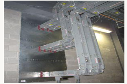
PASS — Sealed Penetration Firestopping electrical conduit penetration through fire-rated wall — sealed correctly
