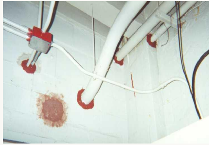
PASS — Listed Firestop Listed UL firestop system at conduit penetration — correct F/T-rated assembly
