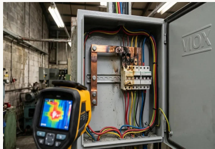
FAIL — Thermal Damage Thermal damage on busbar — discoloration indicates overheating at connections
